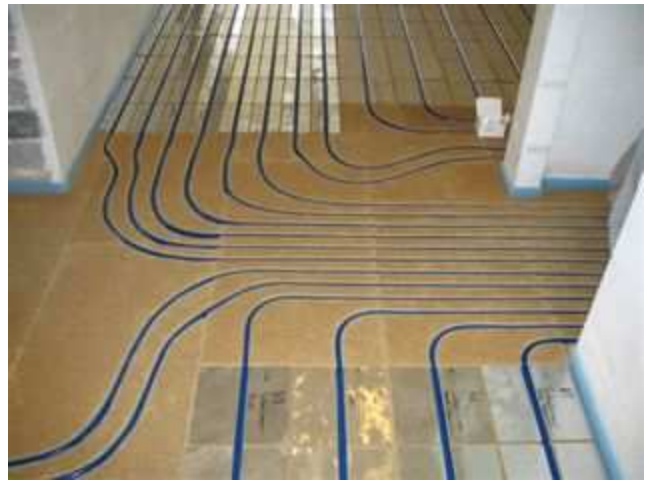
Heating pipes leading from manifold area
