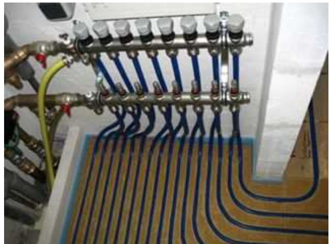
Pipe installation leading from manifold before aluminium diffusion plates are positioned on top
