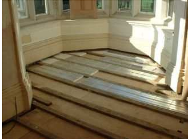
Existing joists battened and lined with ply 30mm below top of joist. IDEAL panels cut to fit tightly between.
