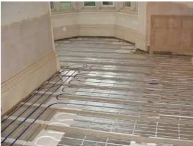
Flow and return pipes as well as circuit pipes channelled through joists.
