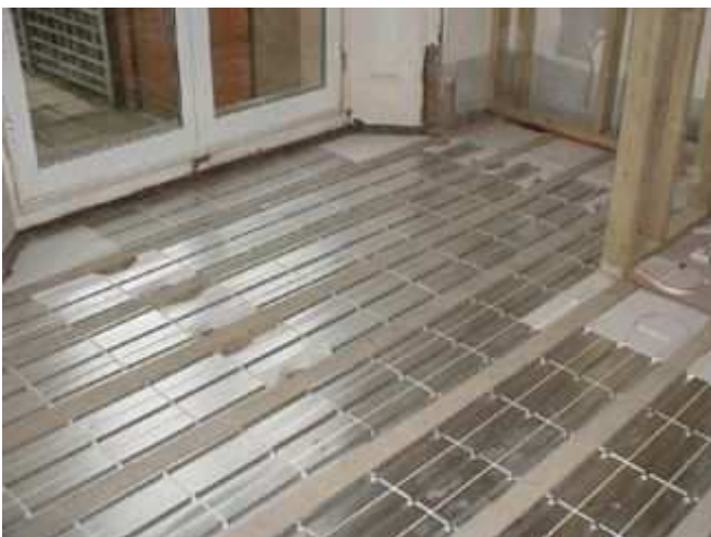
Jupiter Edge Zone (EZ) panels used to provide 3 pipes per joist void.
