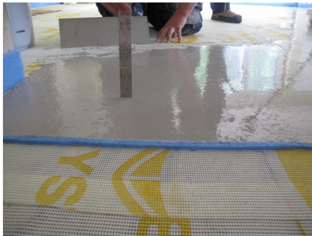
The depth of screed is checked regularly to ensure the desired height is kept. MortaColl is not intended as a levelling compound and will only follow the level of the substrate beneath.
