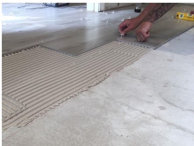
Finally, the finished floor tiles can be installed using standard tile adhesive which conforms to BS EN 12004 Class C2/S1
