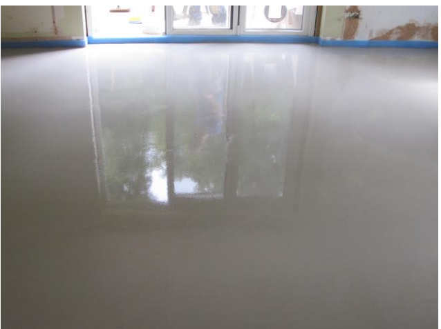
Once completed, the finished screed requires approximately 4 hours to cure before floor finishes can be installed. Expansion joints at thresholds should be observed.
