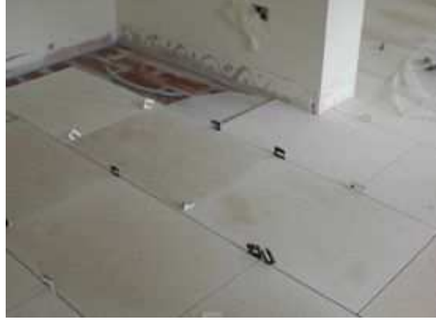
Large format 800 x 600 x 20mm limestone slabs being laid directly on the Screed Replacement Tiles
