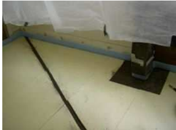
Channels left where insulation is installed up to conduits are filled with pulverised slate ensuring channels remain full and stable
