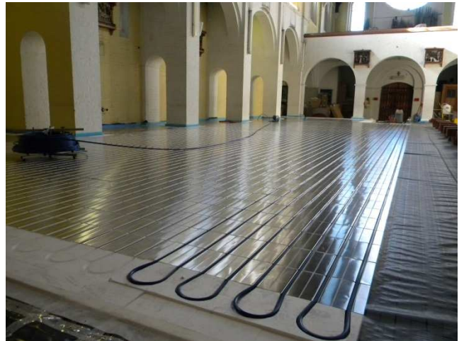
The JUPITER heating panels were then installed rapidly followed by the heating pipe work.
