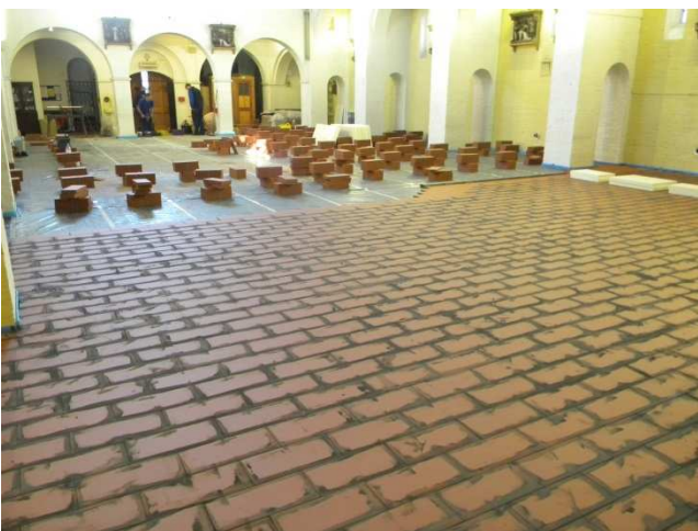
Once the heating was installed, the system was covered with a slip membrane and then tiles with the Screed Replacement Tile
