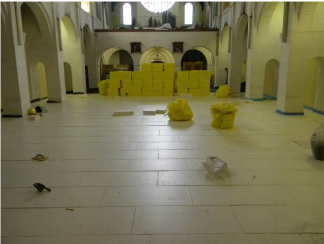
Following the installation of a damp proof membrane 120mm rigid insulation was loose laid.
