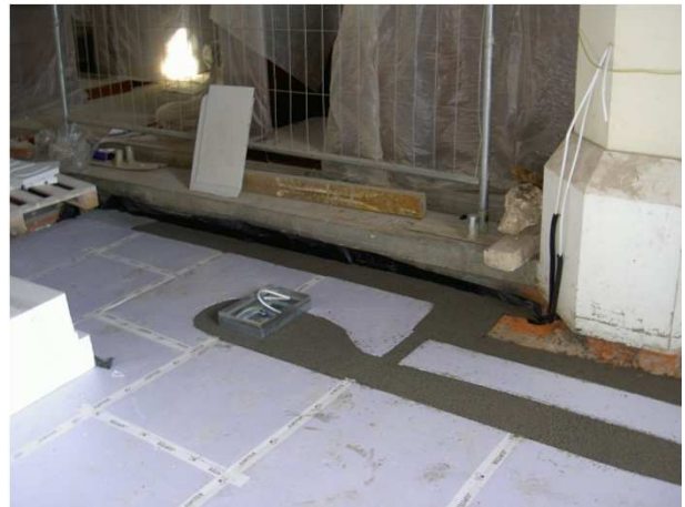
Channels cut in within primary insulation for electrical services. In filled with granulated levelling slate. Sunken floor box shown in situ.
