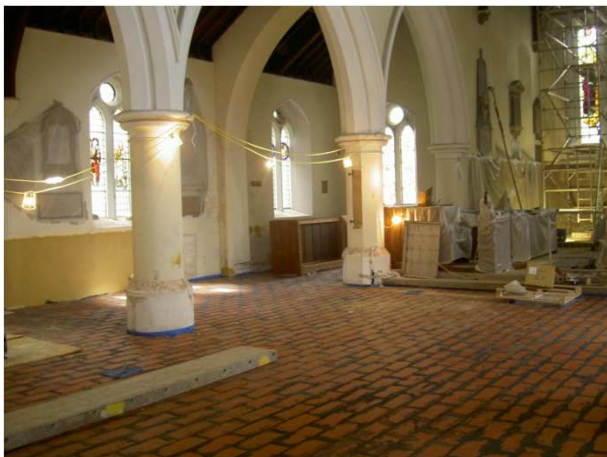
Screed Replacement Tiles installed in preparation for carpet and natural slate finish.
